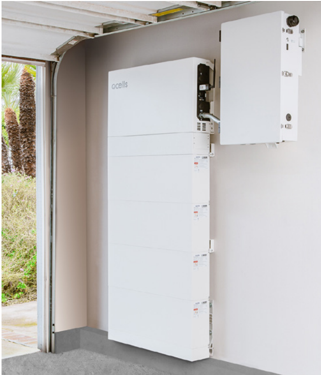
San Diego, CA homeowner installation
